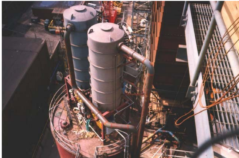
Filter-Receivers on a Silo roof
